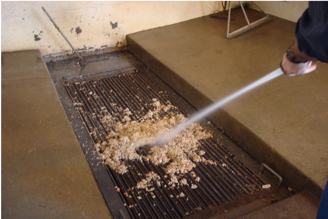
Figure 2.7. Ram's Horn Food Waste Being Sent Through the DWRF Septage Receiving Facility Bar Screen
