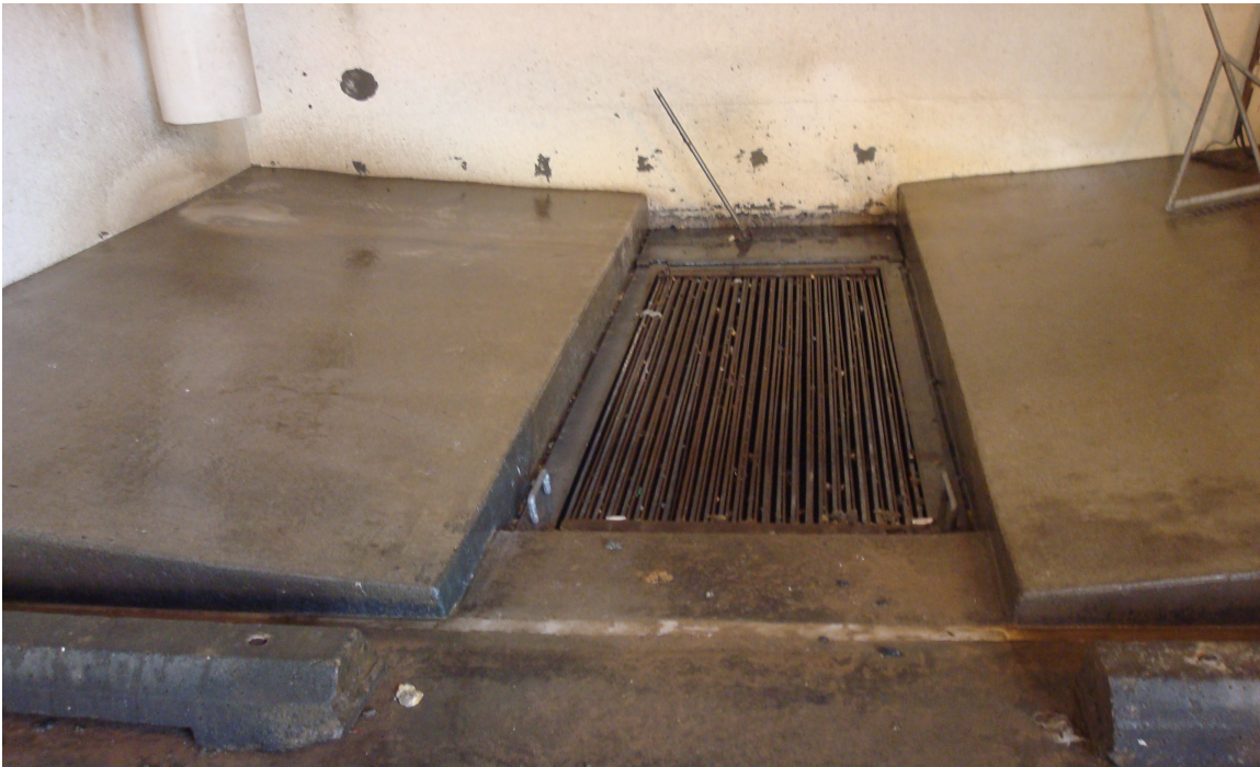
Figure 2.2. Picture of DWRf Septage Receiving Facility Bar Screen
